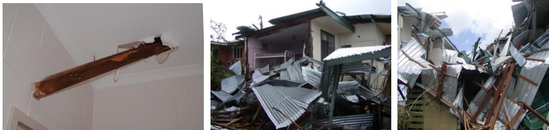
Houses damaged by wind-borne debris during TC Larry (Innisfail, Qld, 2006)
