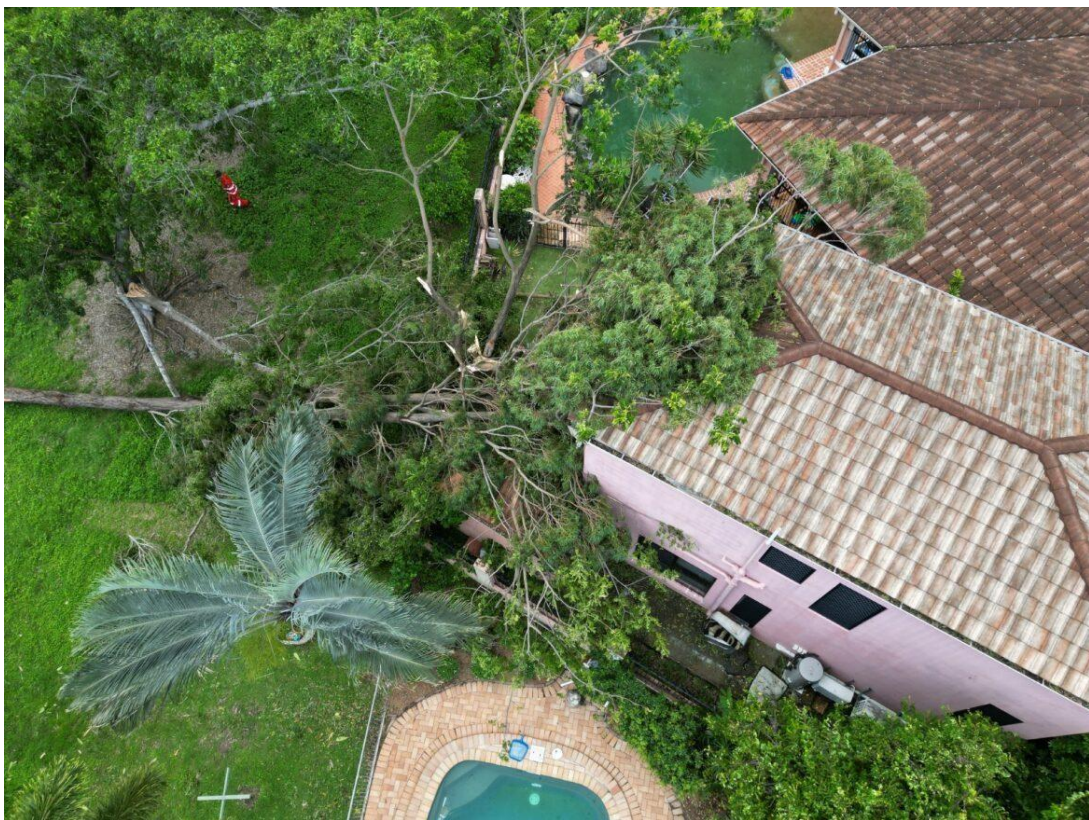
Image 1. Vegetation causing structural damage post Tropical Cyclone Kirrily - Townsville Source: SES
